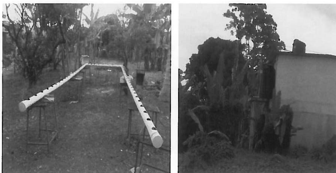
Photo: Installed water tank (right) and pre-installed irrigation system (left) – School in Trelawny
